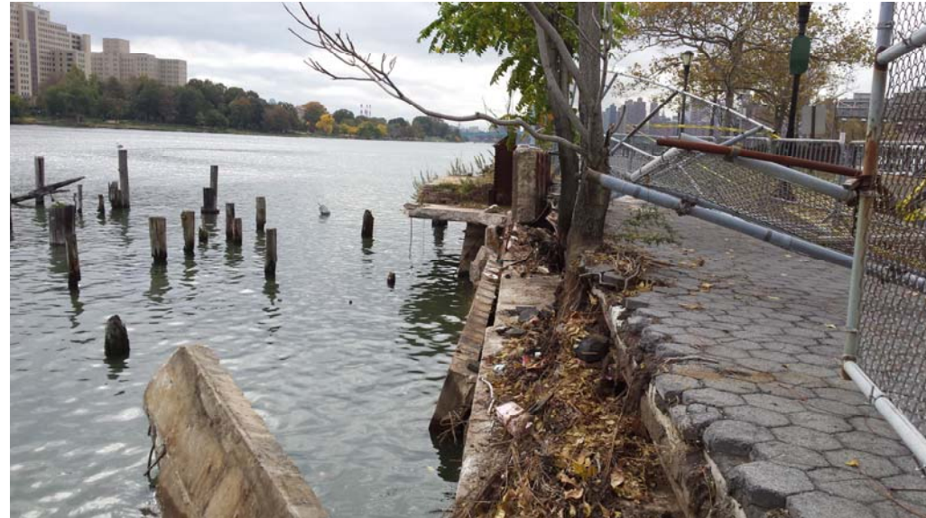
Partial collapse and loss of bulkhead
